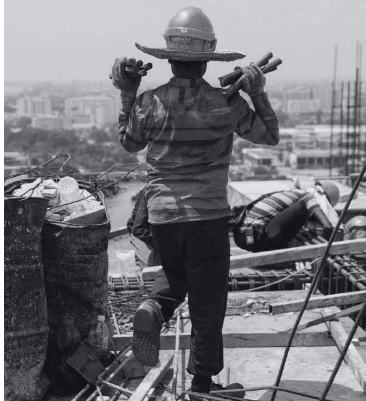
Rohingya workers employed on a construction site in Penang. Construction sites, which are numerous in Malaysia, are one of the few ways the Rohingya can earn a living in the informal economy, but some employers take advantage of their irregular legal status to deprive them of their full wages. (Penang, Malaysia, Apr 2019) | © Arnaud Finistre
