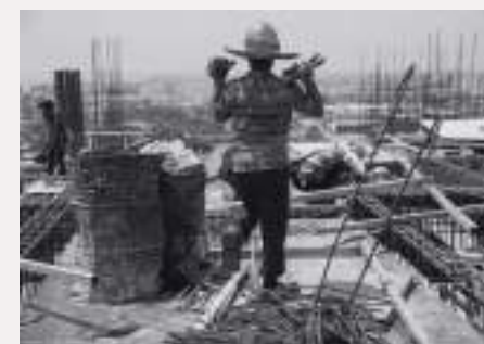
Page: 22 Copyright: Arnaud Finistre Description: Rohingya workers employed on a construction site in Penang. Around half of the workers on the site are Rohingya, who, with no legal status in Malaysia, are not legally allowed to work. The other workers are Bangladeshi, Indian, Indonesian or Malaysian. Rohingya workers often work in particularly precarious safety conditions, frequently sleeping on site in basic shelters to save money. This allows them to send money to their families who have stayed in Myanmar or who have fled to Bangladesh. Some unscrupulous employers take advantage of their irregular legal status to deprive them of their full wages. Construction sites, which are numerous in Malaysia, are one of the few ways the Rohingya can earn a living in the informal economy, but many workers have been cheated out of their earnings. Penang
